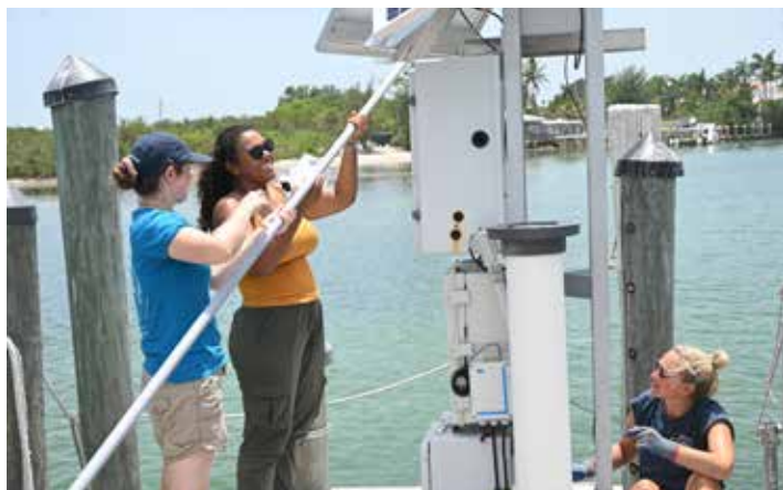
Katy Holmes, intern Ana Fernandes Costa, and Cecilia Thompson install a hydrophone in a protective pipe sleeve at the SBLN's station in New Pass.
