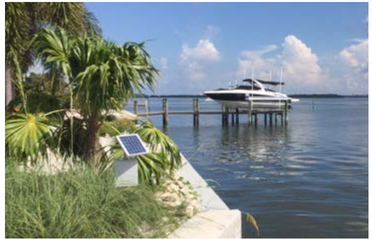
Fig. 2 Solar-powered stand-alone receiving system on Longboat Key.
